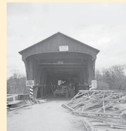
Bailey trusses, a type of portable prefabricated bridge, were added to the structure in 1959.
