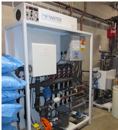
Figure 1 water recovery system
