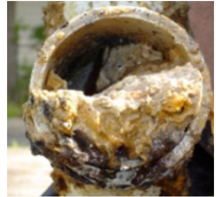
Blocked wastewater pipe
