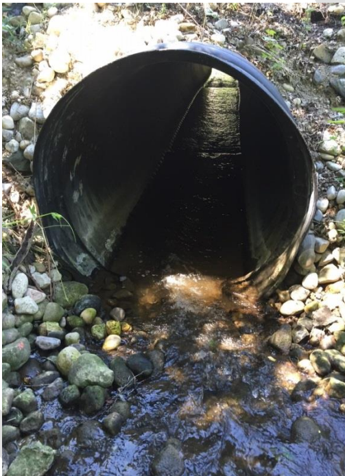
RD-ST1 Structure Inlet
