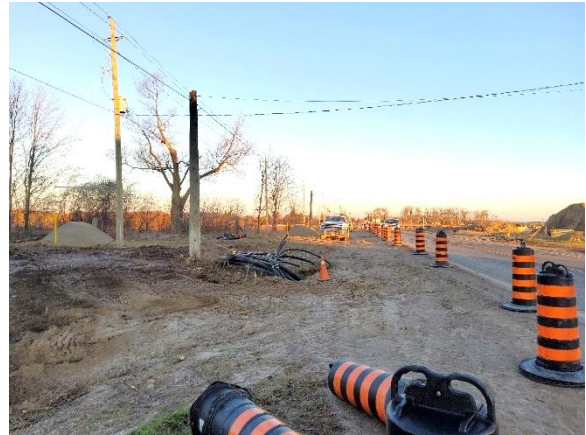
Image 3: Previous disturbance caused by utility installation and recent tree removal; no potential.
